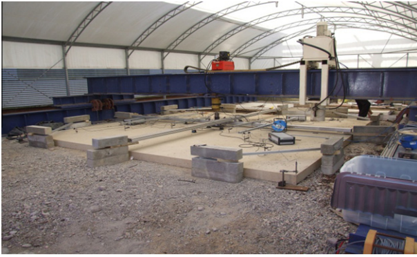
Fig. 1. Ground slab facilities at the University of Greenwich – 2nd test series in progress.
